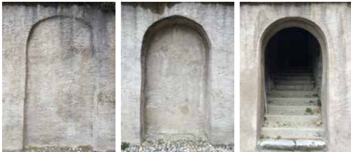
Repetition and variation: arches and staircase in retaining wall/ Herhaling en variatie: bogen en trap in de keermuur, Casima, Val di Muggio, Ticino
